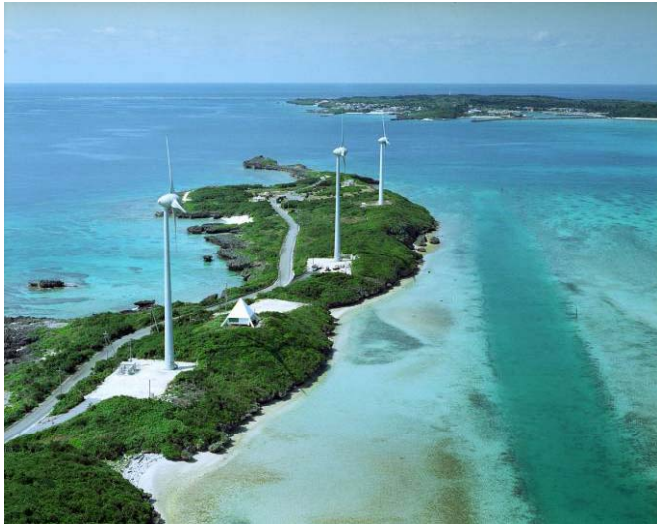
Existing Wind Turbine Generation
