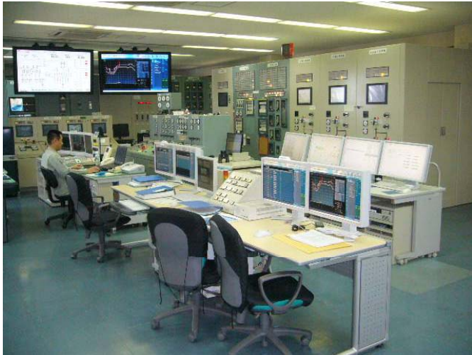
Central control room of Miyako No.2 Power Station
