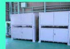
Grid connecting battery system development
