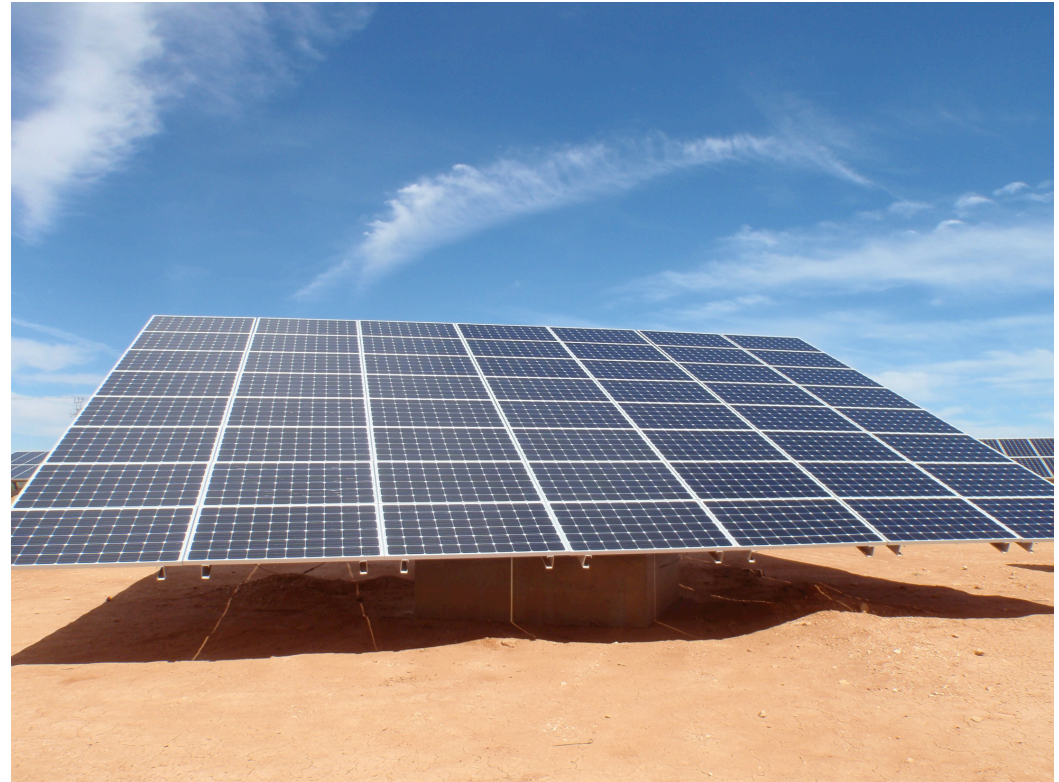
EMC Solar Farm, Carnarvon
