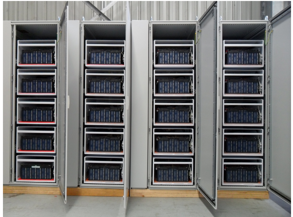
8MJ Storage Capacitor Bank – 20 * Modules – 960 * Capacitors
