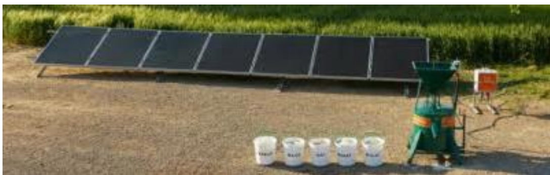
Figure 3 - A 1kW battery-free "direct drive" solar milling system
