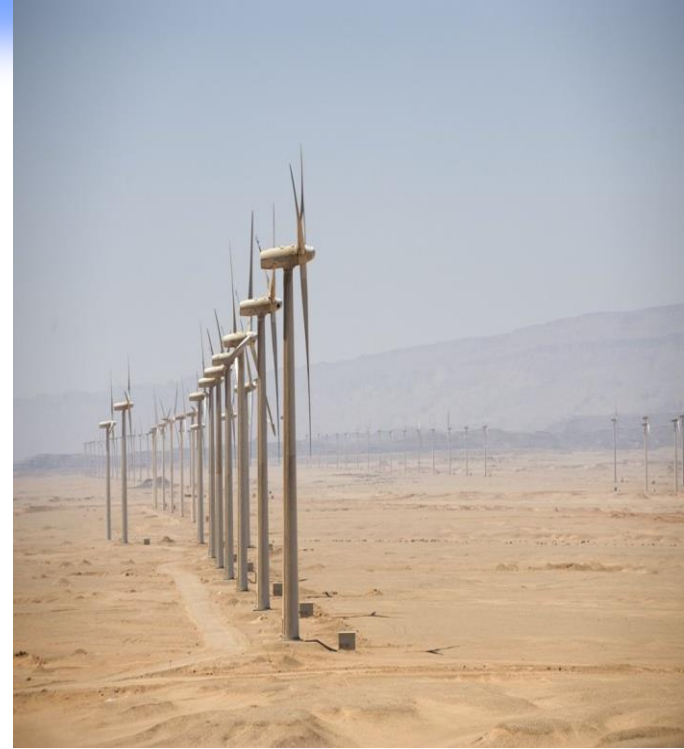
Zafarana Wind Farm, Egypt
