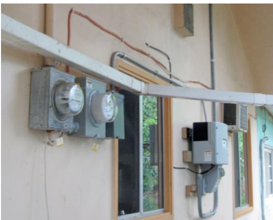
Inverter and meters
