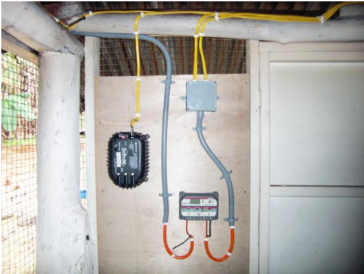
Panel connection box, charge controller and inverter
