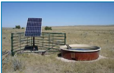
Solar water pump 2-4kW for irrigation (9x4x5x4 = 720W shown)
