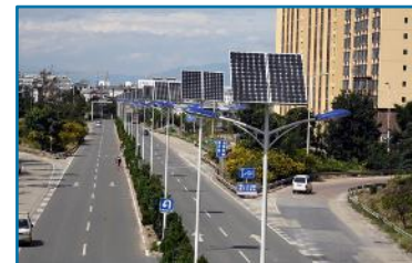
Solar street lights 100-200W for minor roads (360x2 = 720W shown)
