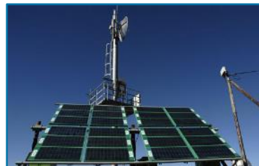
Communication mast 1-6kW depending on use (180x24 = 4,320W shown)
