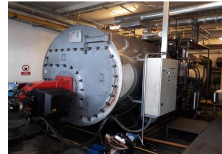
Fossil fuel Boiler to generate steam
