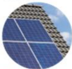
Solar home systems
