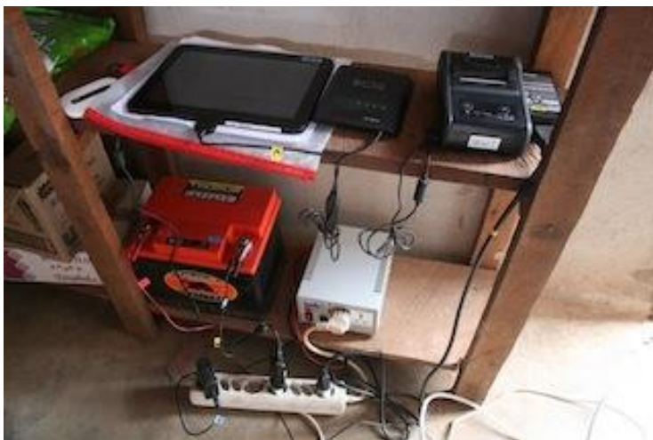
Equipment charged by solar panel
