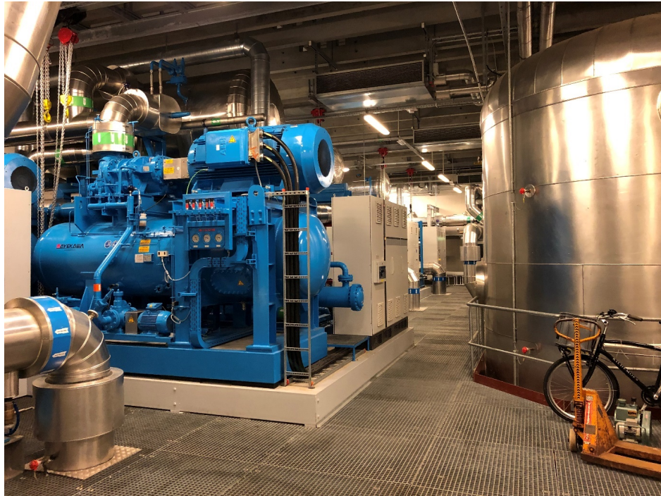
HOFOR's District Cooling Plant in Adelgade Copenhagen – sea water free cooling and compressor cooling. The system is operated at delivery temperature 6 oC and return temperature 16 oC.
