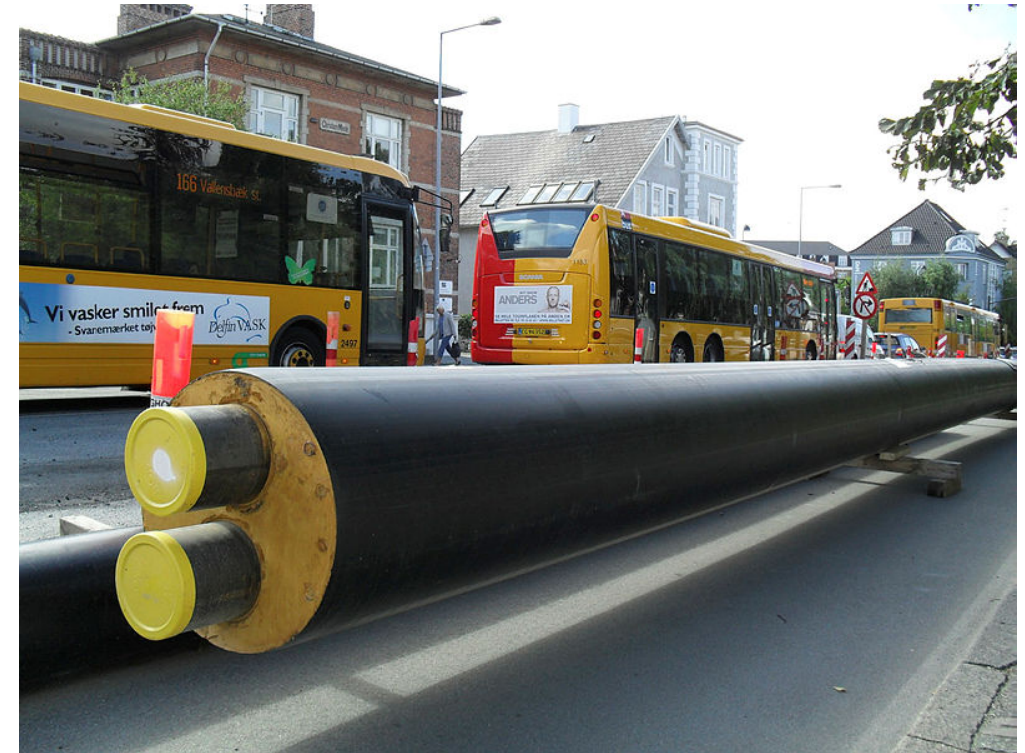
District heating pipes in Gentofte, Denmark
