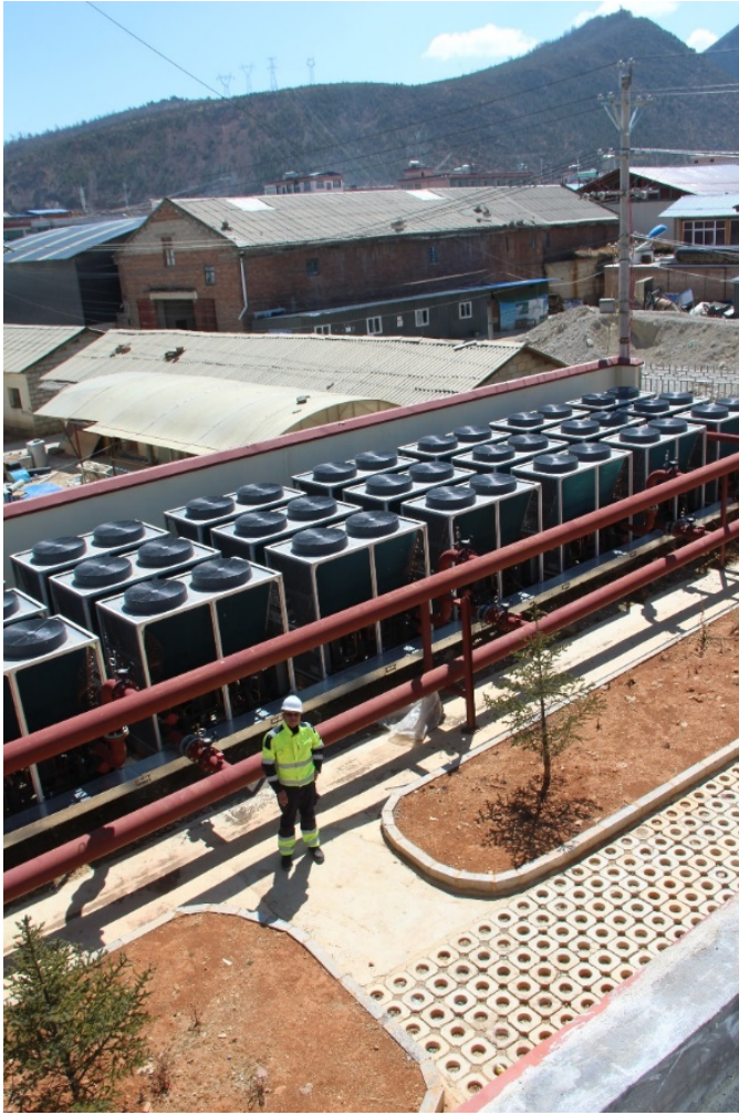
View of heat air-water heat pumps in the year of Shangri-La Boiler House No. 5. Photo: Shangri-La. 2018 03 13, Andrew Christensen, COWI A/S.
