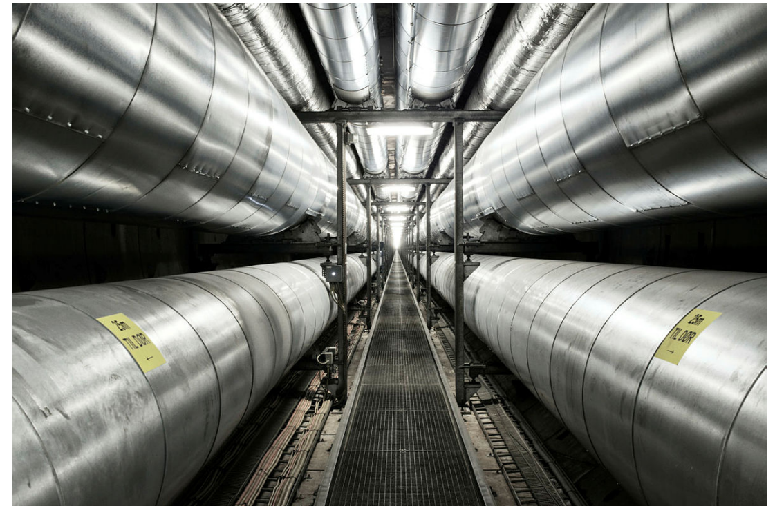
District heating tunnel under the Copenhagen Harbour Two sets of forward and return pipes
