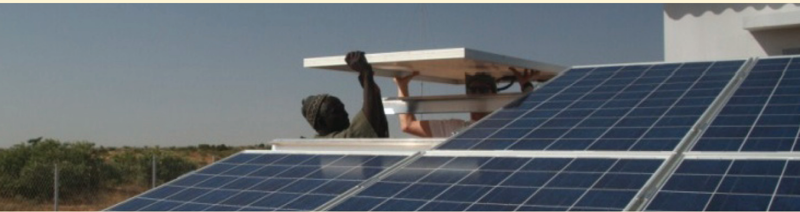
Installation of solar panels in the village of Sine Moussa Abdou, Senegal Courtesy of INENSUS West Africa S.A.R.L
