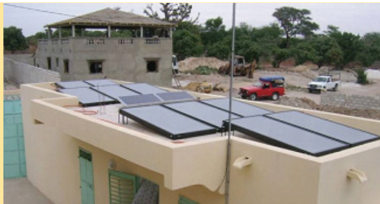
Solar Water Heater in rural area in Senegal Courtesy of Enersol
