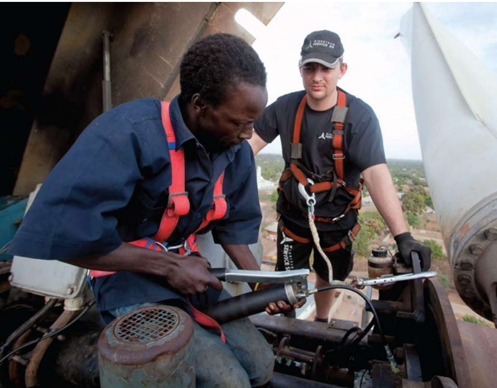
Maintenance work in progress at the Batokunku wind energy plant in The Gambia Photo: M. Kottmeier Source: www.rural21.com
