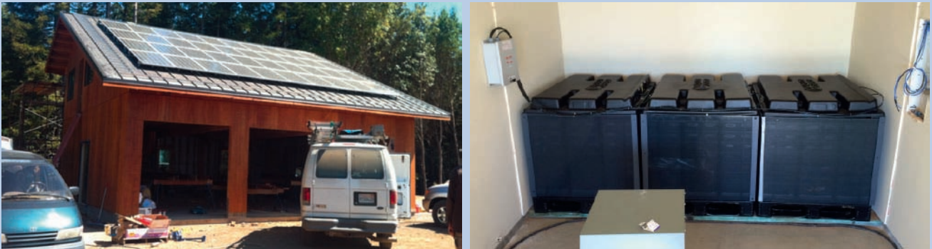
Solar PV power generation (left) coupled to aqueous hybrid ion battery storage pack by Aquion Energy (right).
