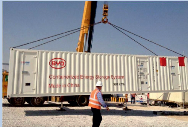
Containerised energy storage system by BYD.
