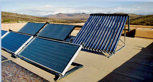
Figure 2: Flat-plate solar collectors (left) and evacuated tube collectors (right) installed on a single roof
