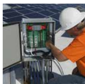
Cabling and grid connection
