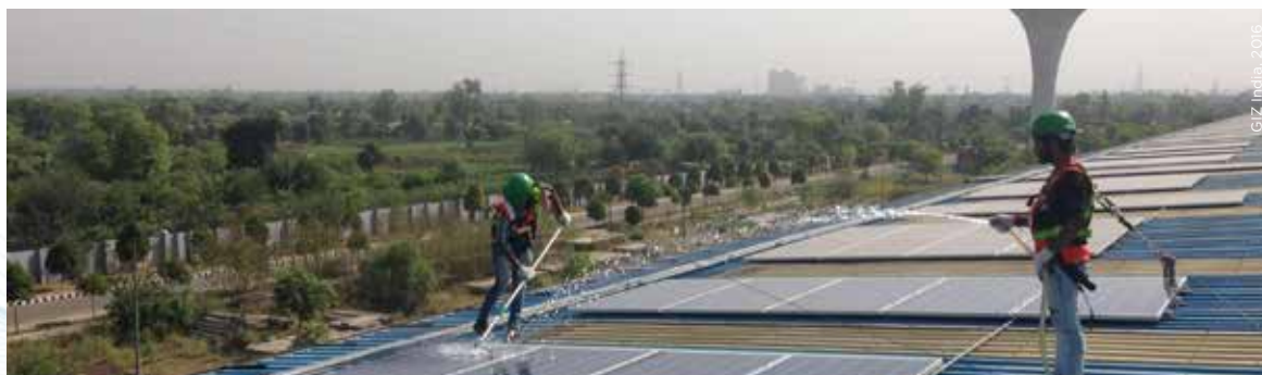
The Delhi Metro by 2017 had commissioned solar rooftop systems with 20 megawatts-peak capacity
