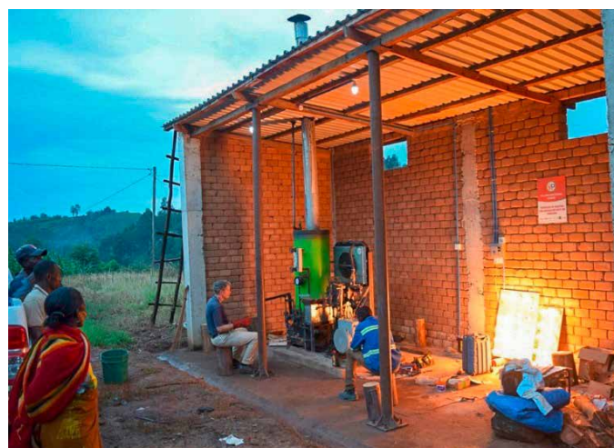
VIP's heat and power generation
