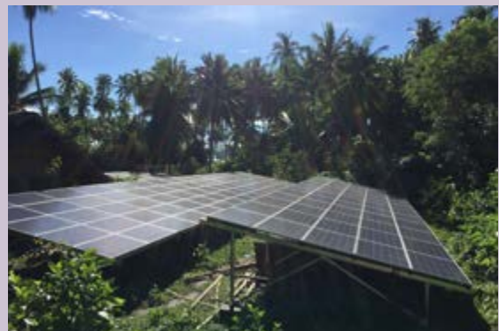
Solar power plant in Qi Palawan, a resort in the Philippines
