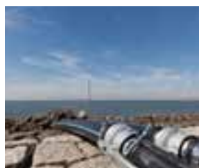
Cabling and grid connection
