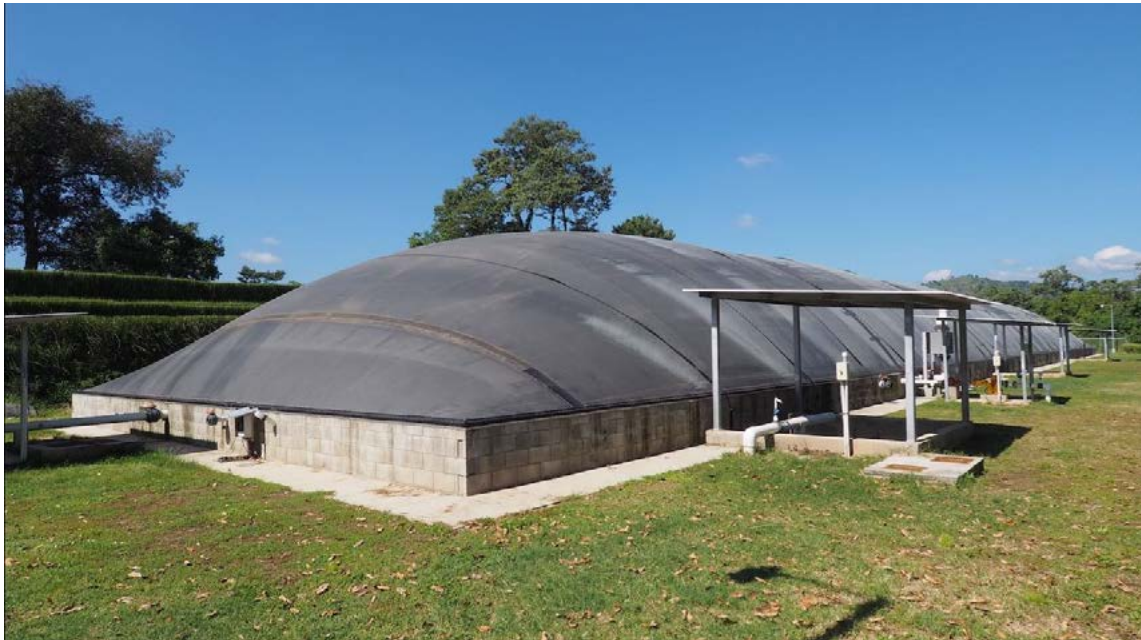
FIGURE 6: Covered lagoon digester
