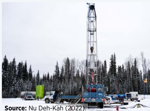
Photograph 2 Geothermal site of the Tu Deh-Kah project, in Canada
