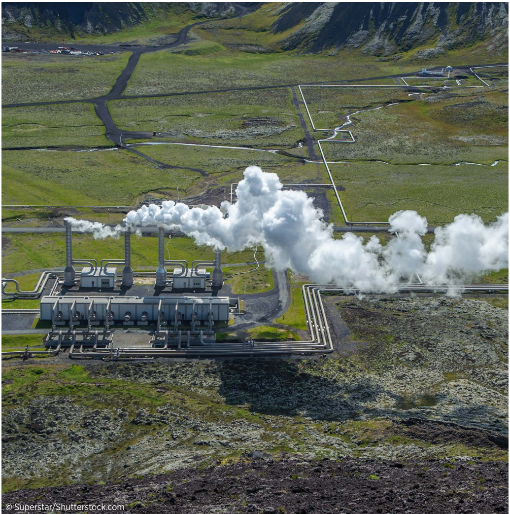
Geothermal power station in Iceland.
